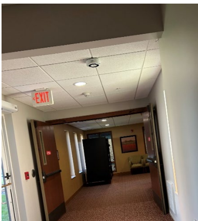
Connection number one to nursing facility
