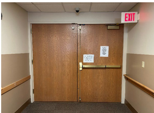
Fire doors that separate the settings
